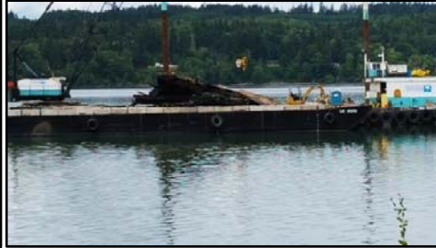
A large portion of the Former Log Transfer Facility, on a barge heading for disposal.
