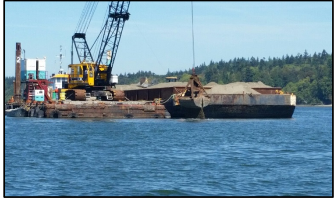
Barge and crane placing clean capping material in the central part of the bay (SMA-3).
