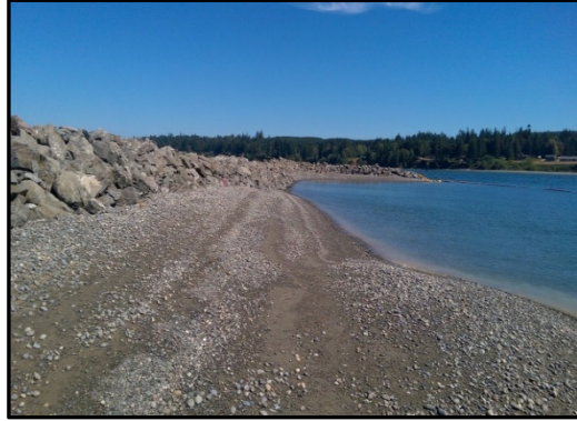
After: SMA-1 intertidal area with piles pulled and capped with clean material
