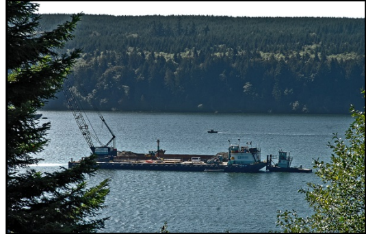
Barge and crane placing clean capping material in SMA-3. Photo courtesy of Terry Moyemont.
