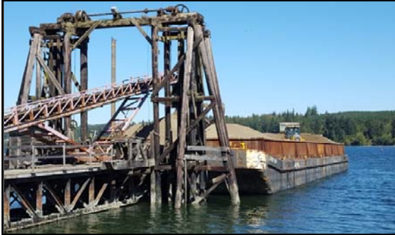
Clean capping material being loaded onto a barge for placement in SMA-3.
